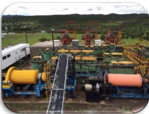
Figure 2 - Andes Processing Mill Facility
